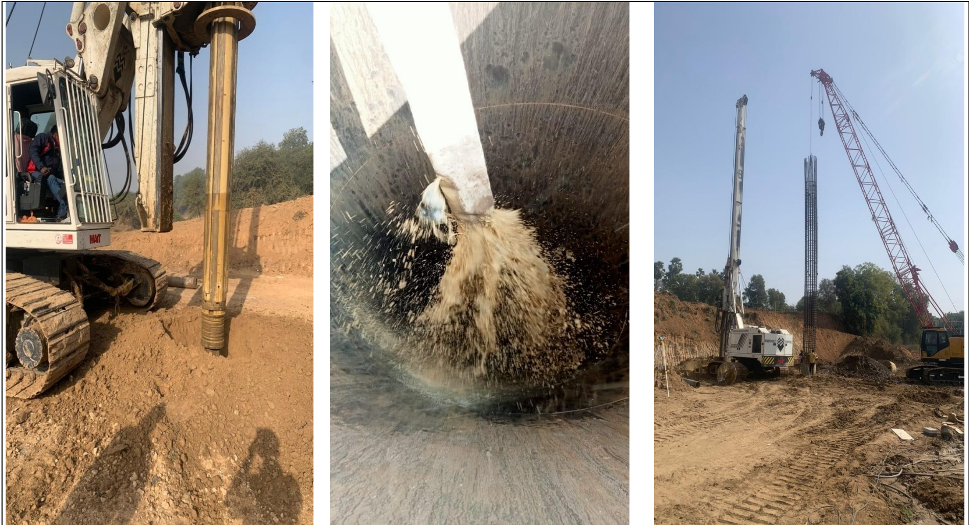
Pile Boring, Applying bentonite and Cage Lowering for Pile of Major Bridge
