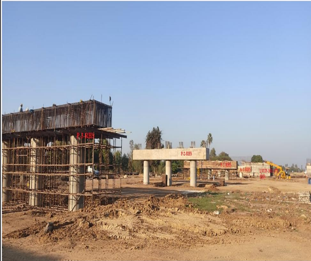
Pier Cap –P-3 reinforcement fixing & Pier Cap A1,P1,P2, RHS A-1 side MJB @ 352+281
